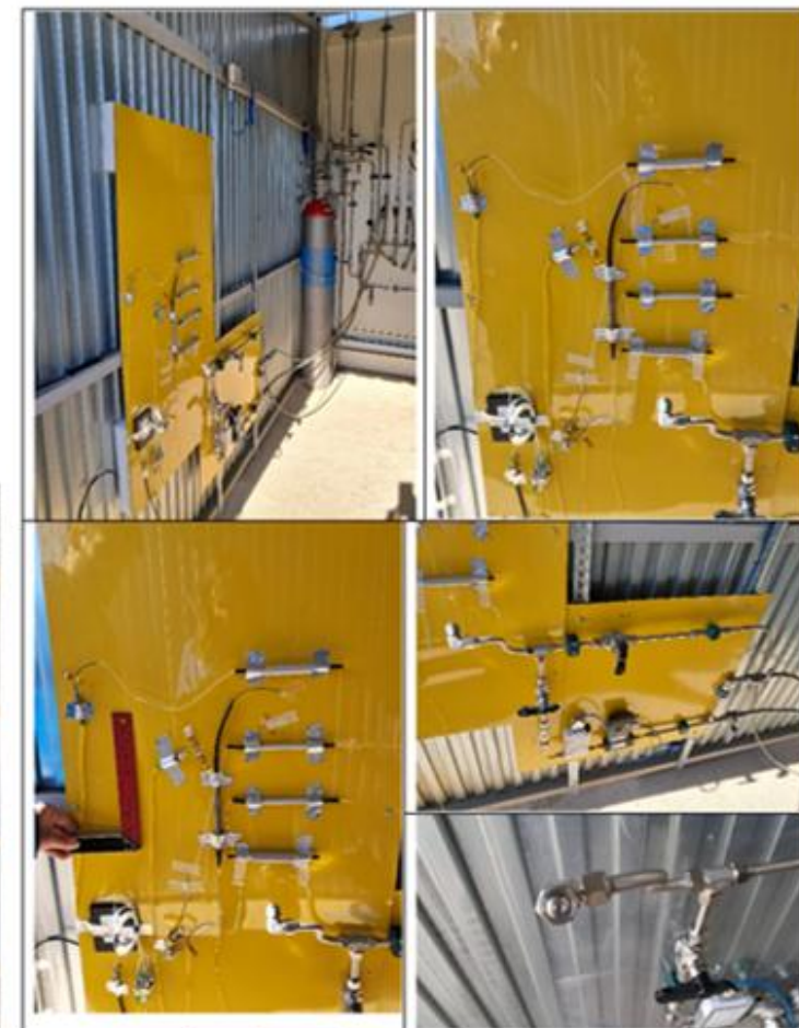
Hydrogen refueling station
