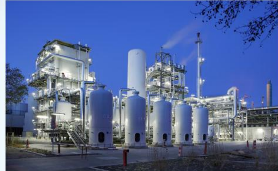
Pressure swing adsorption plant (PSA) (© Linde)
